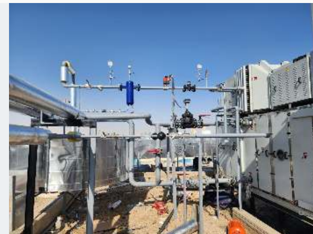
Associated pipework and valves
